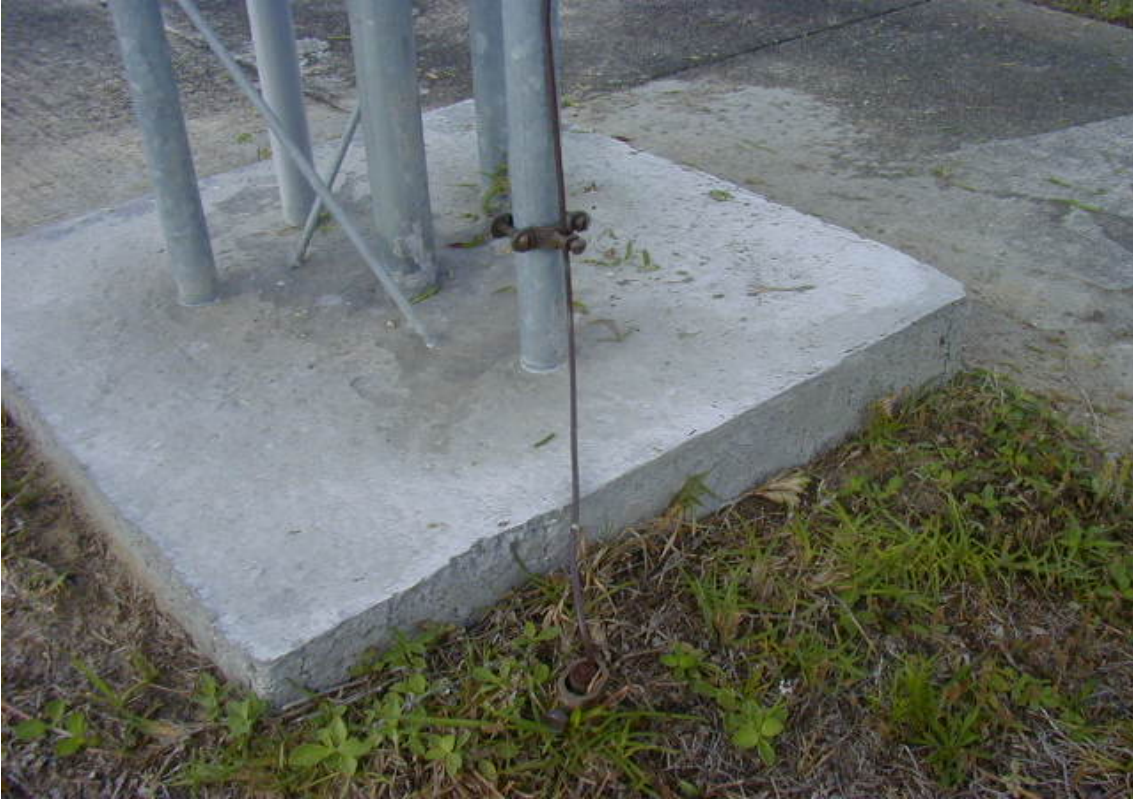
Illustration – Ground wire connected to Tower
